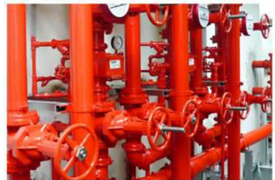
a structure for Application - Fire Fighting
